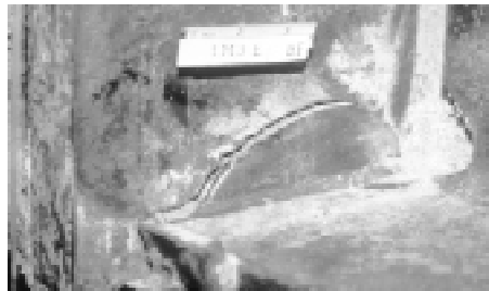
Figure 1 Divot Failure in Column Flange
